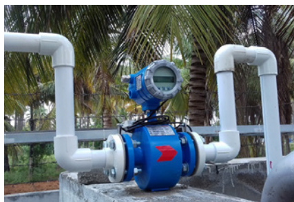
Flow meter installed at all raw water input points for enhanced monitoring
